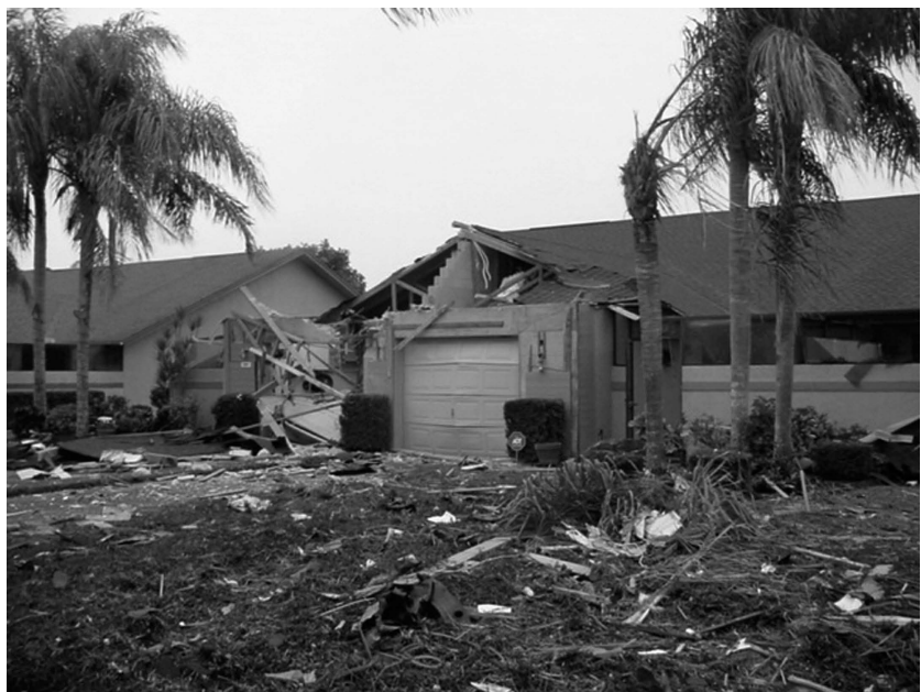
Figure 8.8 First impact in the roof of the house.
